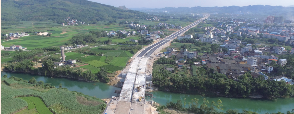
Road reconstruction project connecting Shatang with Shapu in Liuzhou City that is supported by Guangxi Branch
